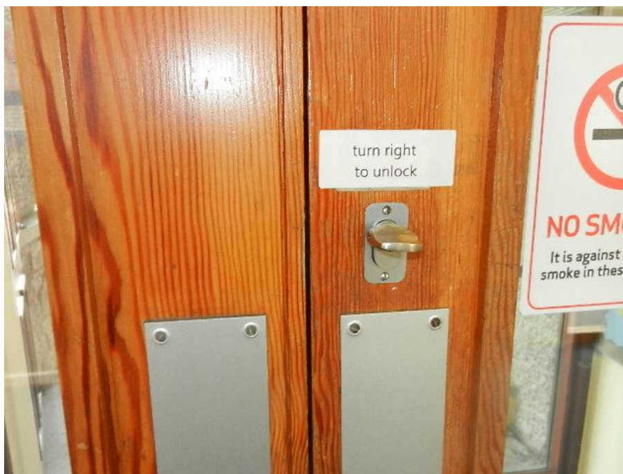
Figure 16: Small thumb turn lock on lobby exit door.
